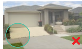
Driveway doesn't align with crossover
