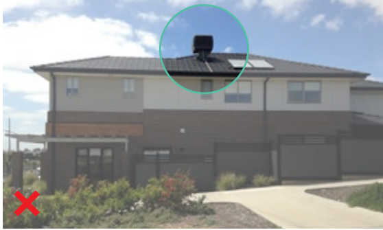
Non compliant evaporative cooler unit above roof ridgeline
