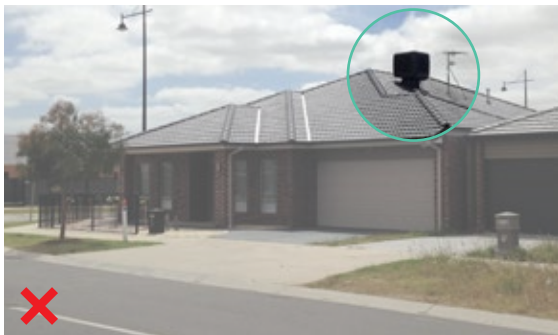
Non compliant evaporative cooler unit located at front of roof
